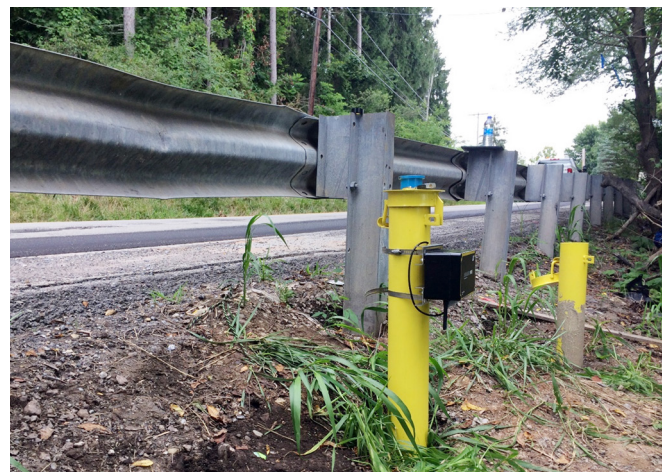
In-place inclinometer installed with datalogger, at the top of slope
