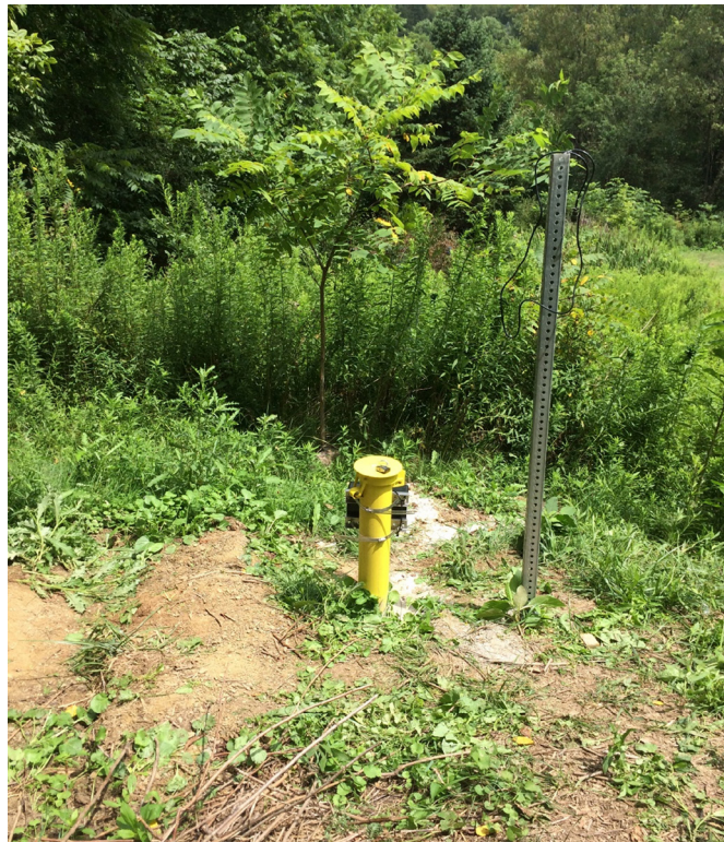
In-place inclinometer installed with datalogger, at the toe of slope
